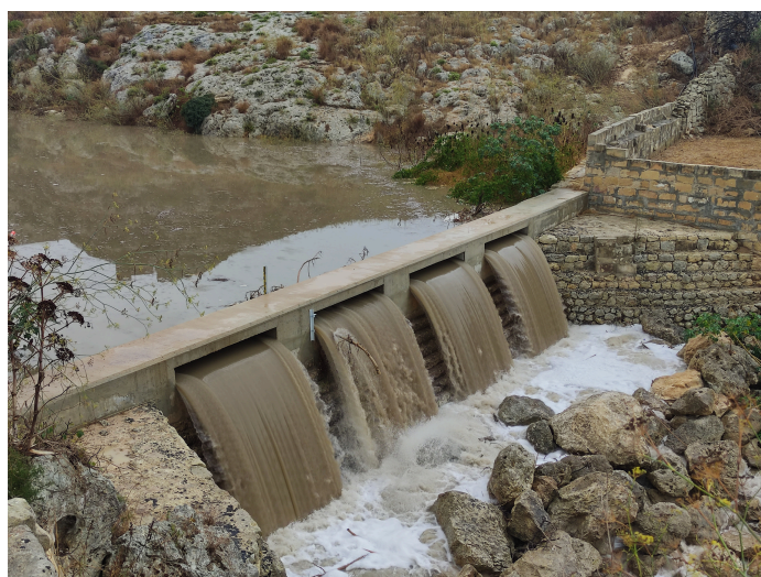
Wied il- Għasel, basin 0 discharge gauging point during the precipitation event of August 30 th 2023
