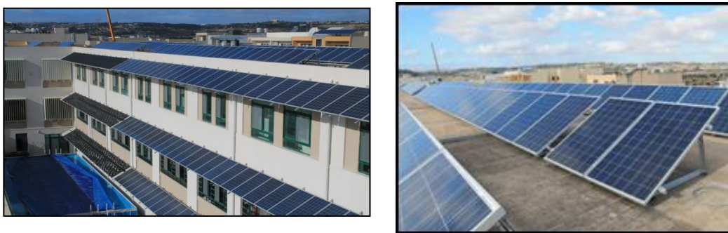
Figure 2: Unglazed pool solar thermal system and PV overhangs on the south courtyard facade (left image) and roof mounted Photovoltaics (right image)
