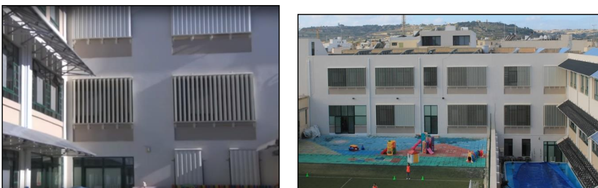
Figure 3: BMS controlled movable external vertical louvers on the East and west facades
