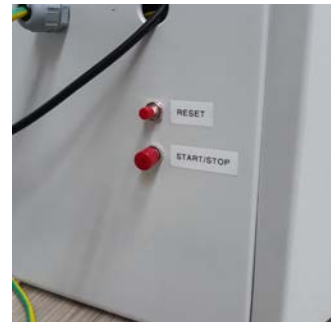
Figure 6.27: Panel Mount Start/Stop Push Button Switch on the Buck Converter
