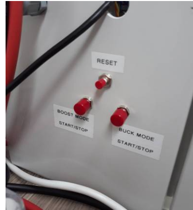
Figure 6.55: Panel Mount Start/Stop Push Button Switches on the Bidirectional Converter
