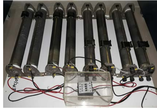
Figure 6.61: Resistive Load Bank
