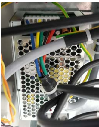
Figure 6.39: Integrated Power Designs DC4-70-4005 - Supplies the PCBs for the Bidirectional Converter
