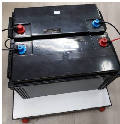
Figure 6.59: 24V 120Ah Battery Bank
