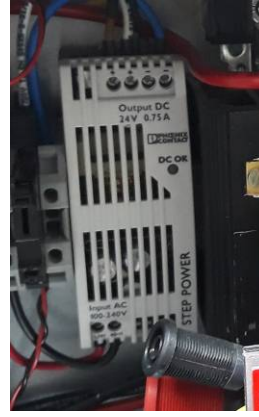
Figure 6.11: Phoenix Contact Step Power 2868622 - Supplies the Contactor Coils and the Heatsink Fan for the Buck Converter
