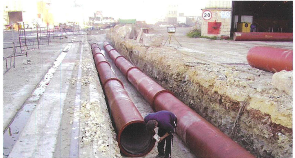
A dual rising-main was constructed to take the pumped sewage from the Marsa Pumping Station into the entrance of the above new gallery.
