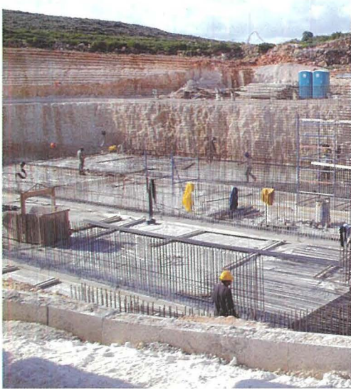
This photo taken during December 2006 shows the construction underway before completion in September 2008 and initial start-up one month later.
