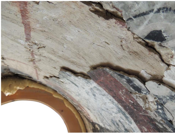
Figure 2. Delamination of the gypsum-based plaster; west apse, Ateni Sioni church, Georgia. © Francesca Piqué, 2012.
