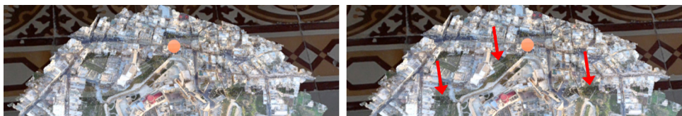
Figure 12: Floor tile pattern visible through darker areas.
