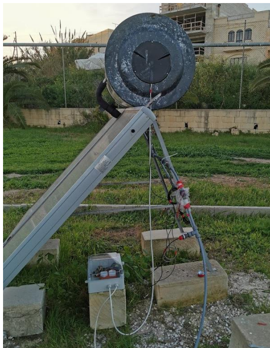
Figure 3.22: Monitoring system prototype installation on a common thermosyphon type SWH, located at the Institute for Sustainable Energy in Marsaxlokk, Malta.
