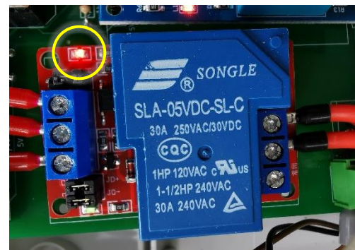
Figure 4.4: UI displaying an 'ON' status for the backup heater (left), and the indicator lights showing 'closed position' status on the relay module (right)
