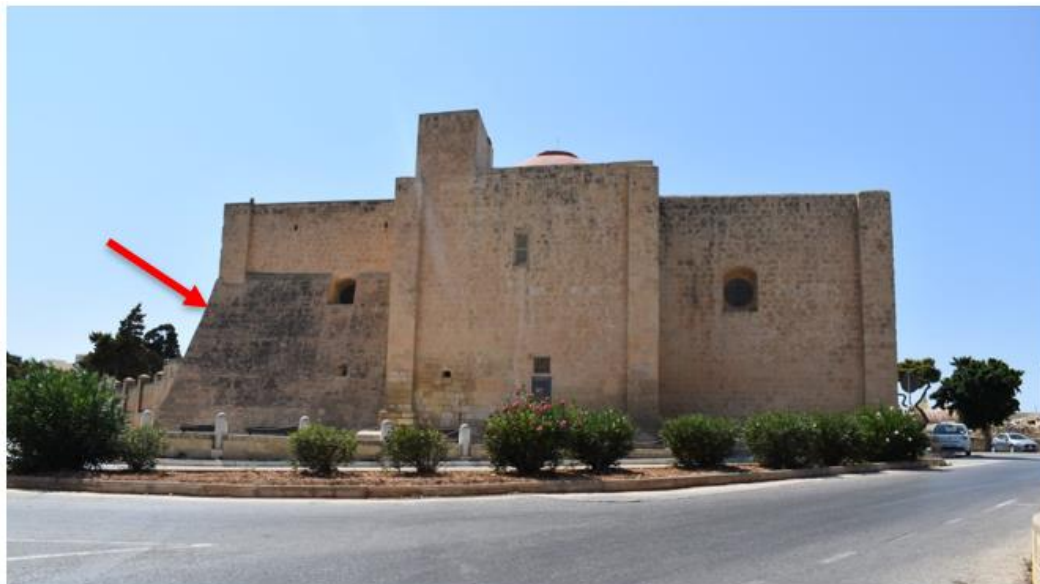
Figure 10. East side of Chapel of San Girgor showing buttress fortification on the south-east side. Photograph by author, October 2020.
