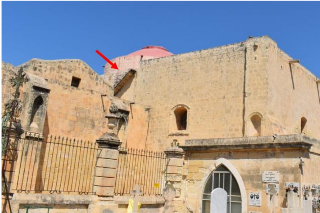
Figure 16. West facing, showing external staircase to roof, Chapel of San Girgor. Photograph by author, October 2020.
