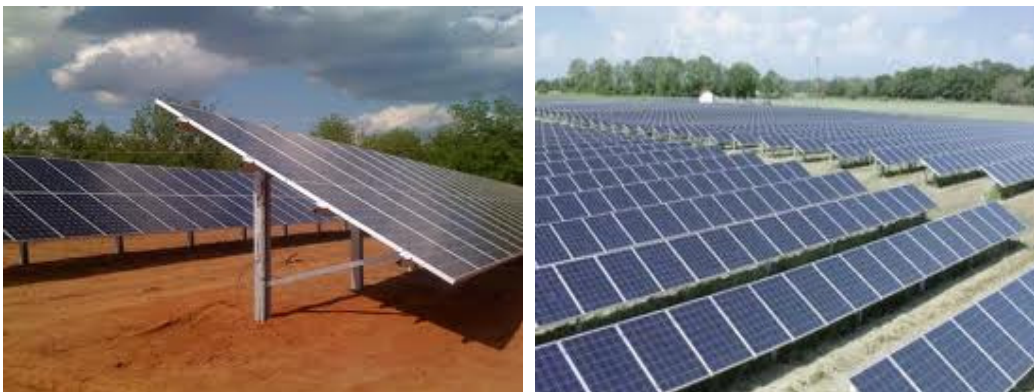
Figure 13: Examples of fixed systems
