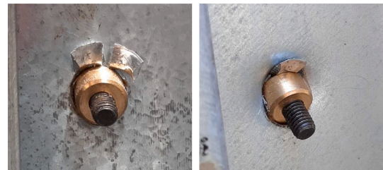
Fig. 20. Failure of the Type 4 connector - failure of the four locking segments followed by the bevelled nut pulling into the CFS sheet.
