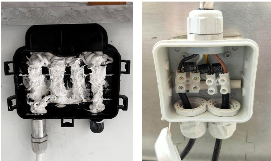
Figure 88: Sealed internal junction box (left) and new external junction box (right).
