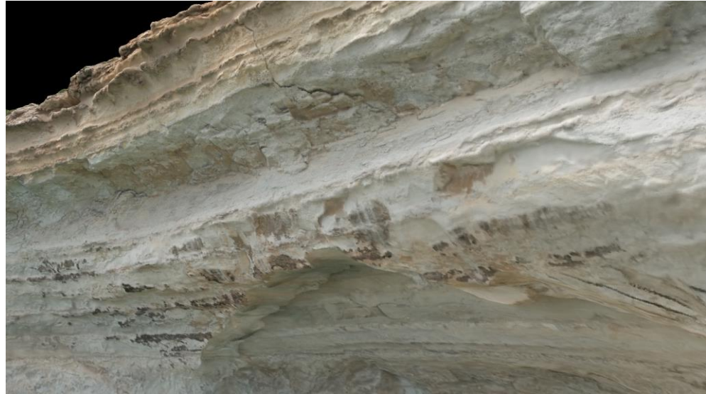
Figure 5. A 3D model render of the crack as it progresses through the Globigerina Limestone. The high-resolution model created allows for monitoring of the shape and dimensions of the crack.
