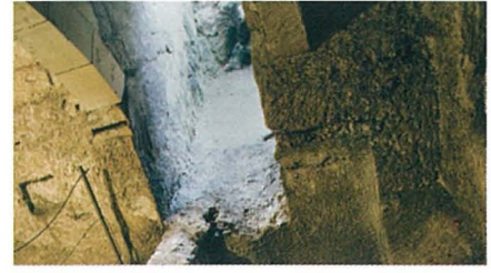
An entrance into another air-raid shelter which underpasses part of St. Paul Street and above which stood a room with a reinforced concrete ceiling for added protection
