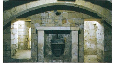
A cauldron that formed part of the central heating system installed in part of the Auberge during the British period
