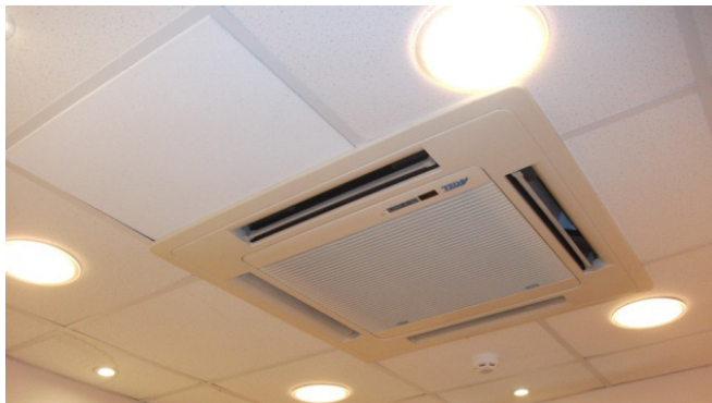
Figure 9.6: Split Type Air Conditioning Units
