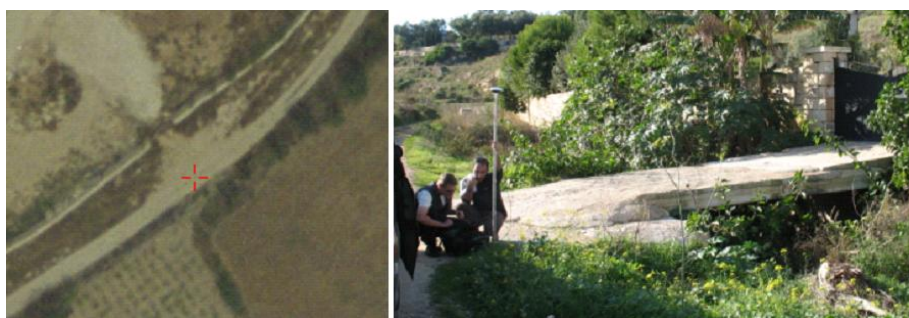
Figure 3: the bridge on the left image is not on the aerial picture
