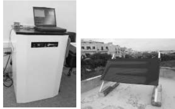
Figure 5. Photographs of the thermodynamic panel placed on the roof and the combined heat pump and storage tank, placed inside the room.
