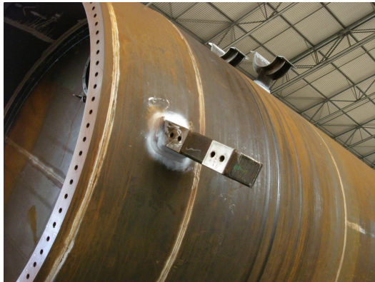
Figure 3: Attachments are welded to the transition piece and the welds are tested using non destructive methods
