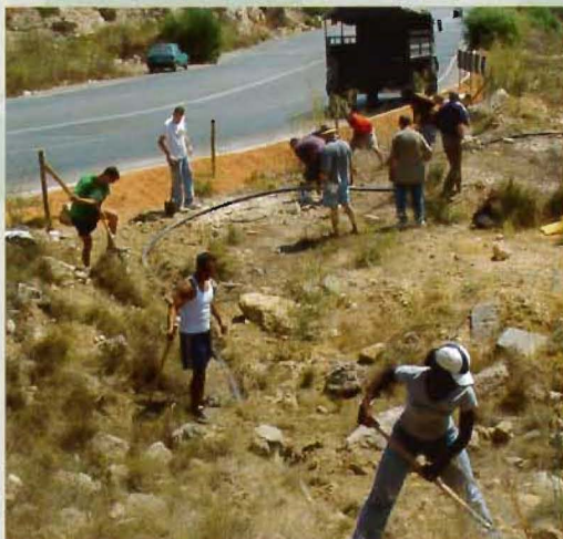
America to the rescue. August. Volunteers from the crew of USS LaSalle help lay the main water feed pipe.
