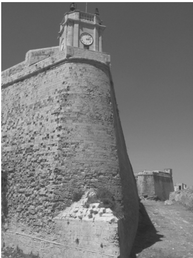
The surviving ditch along the awe-inspiring bastioned ensemble needs to be looked at as an integral part of the Gran Castello. Photo: Kenneth Cassar
