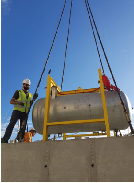
Daniel Buhagiar checking that the FLASC pressure vessel is properly secured to the cement platform
