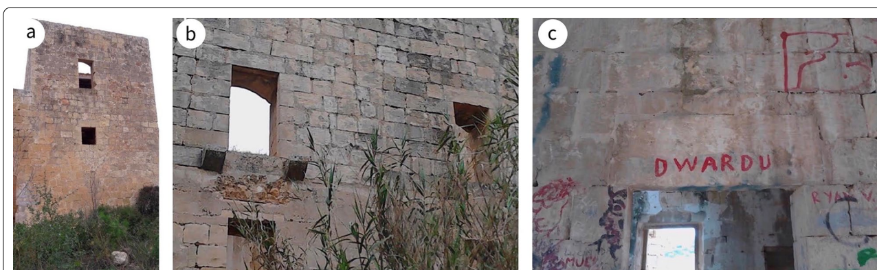
Fig. 10 Masonry lintels: a the lintel could be loaded without failure in tension up to a span \leq 0.9 m; otherwise a relieving arch was introduced, b the stone above the lintel was notched, c depth of lintel increased by 50% the height of a building course
