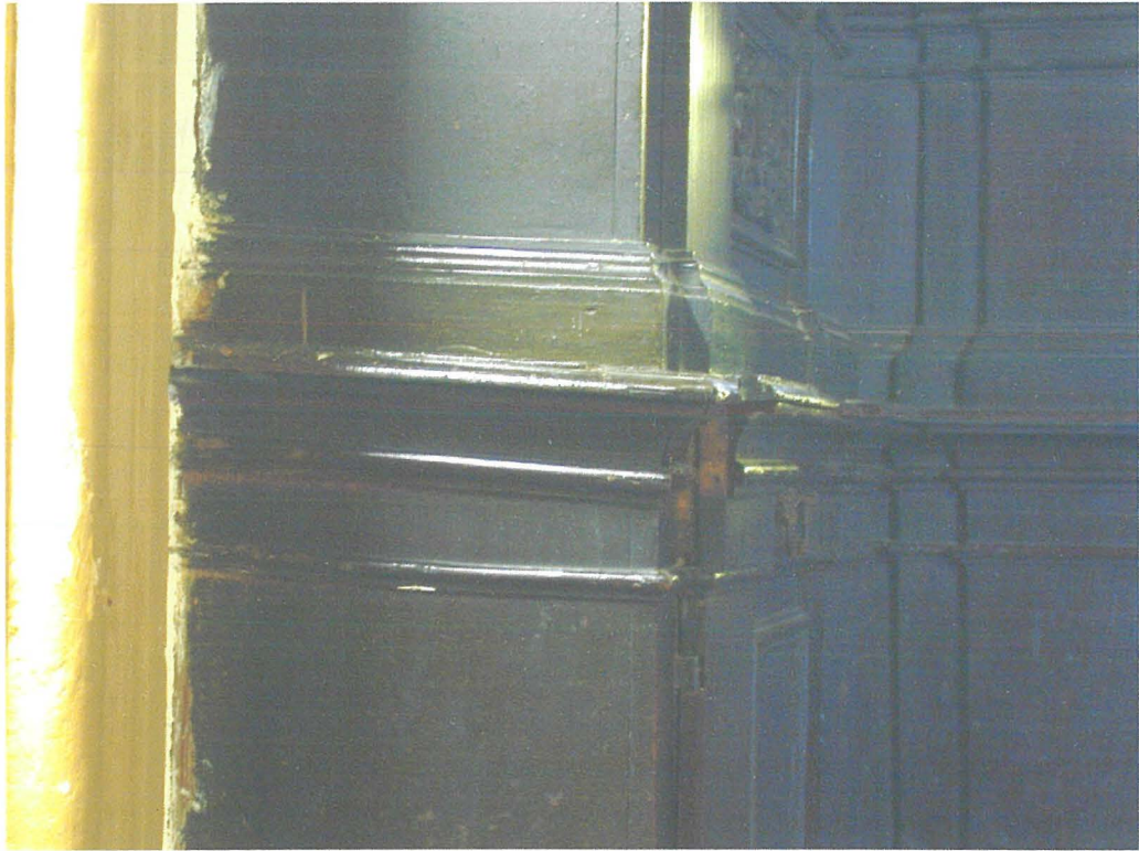
Plate 96 Sacristy furniture sagging due to excessive weight –St Paul’s Church, Valletta
