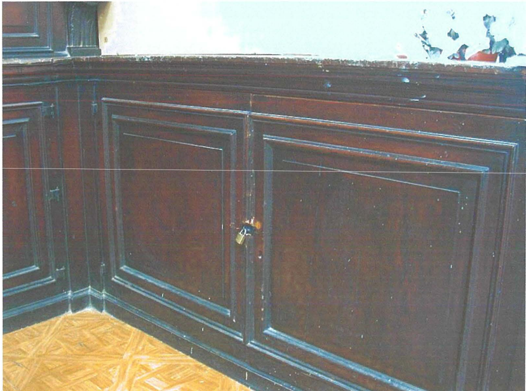
Plate 73 Padlock used to lock two doors, previous intervention – St Dominic's Church, Valletta
