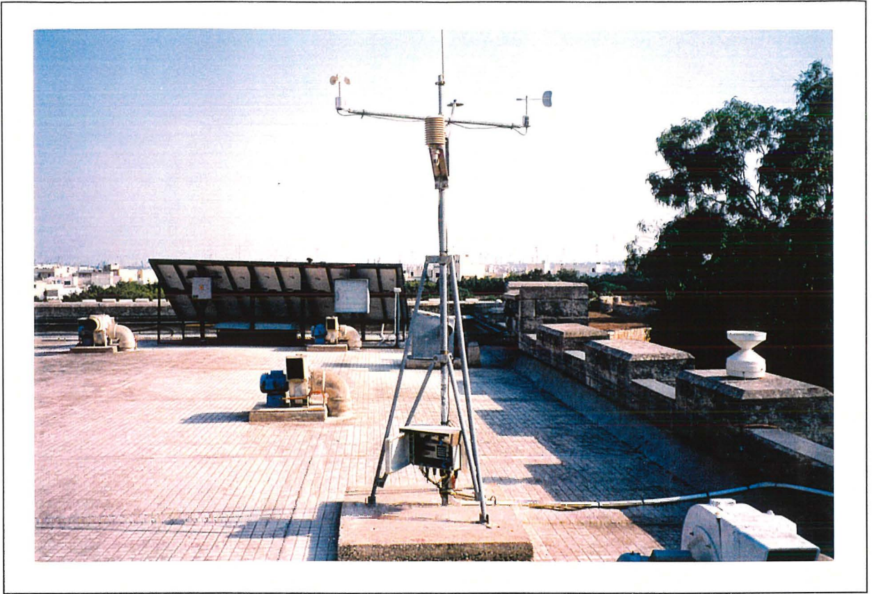
FIGURE 1.8: A photograph of the data-logger and some probes fixed on the weather station. The PV system is seen in the background.
