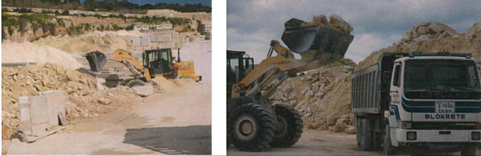
Step 2: Crushing process of the material with jaw then cone then granulator crusher.
