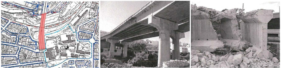
Figure 4.5: Reinforced Concrete elements before and after demolition of the bridge in 2006 Source: MEPA website (plan) and Borg (2008) (photos)
