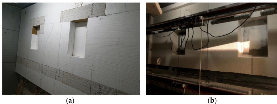
Figure 1. (a) EPS thermal insulation with mineral wool fire barriers; (b) test rig with 4 types of plastering during the test.
