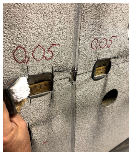
Figure 6. Testing of the bond strength of ETICS: an example of the typical pull-off at the joint of EPS/MW.
