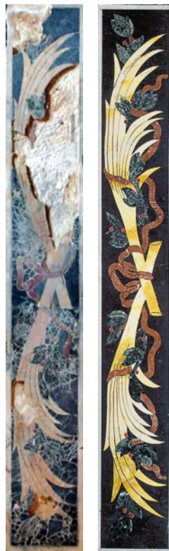
Col.pl. 6a. Detail of floor slab no. 137 to Frà Lucas Bueno (d. 1668) in the nave, St John's Co-Cathedral, Valletta, Malta, here in a ruinous state.
