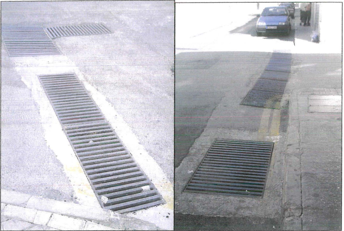
Plates 5.3 and 5.4: Canals made by the B'Kara Local Council for rainwater conservation
