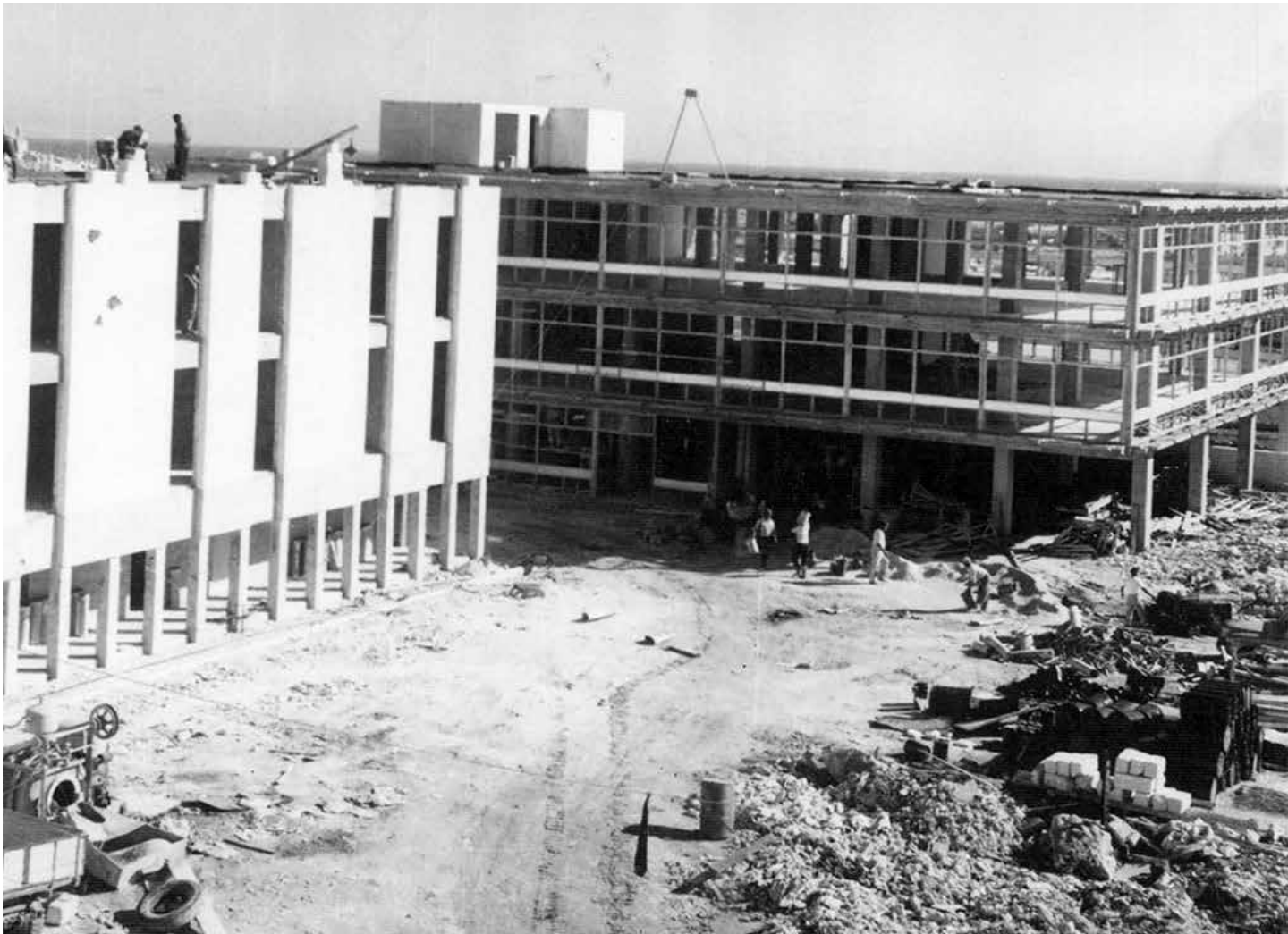
Fig. 10: A partial view of the Humanities building and the Library building under construction
