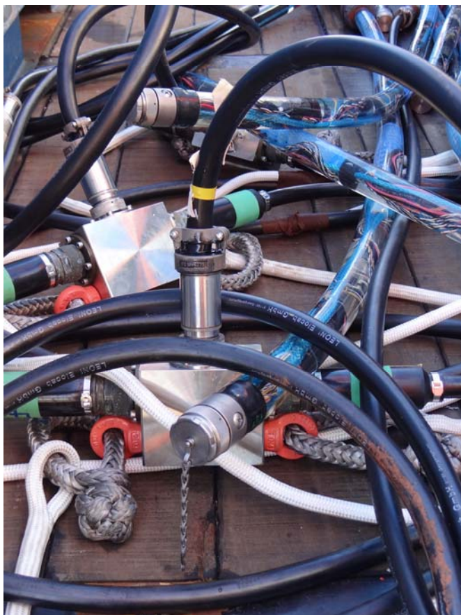
Fig. 21 Photograph of cross cable, drop leads and streamer section during dry test on board.
