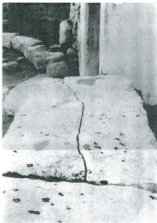
Plate 2 Horizontal block showing a deep crack throughout the entire length. Tarxien Temples.
