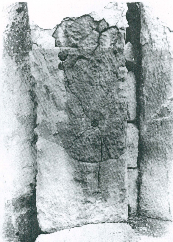
Plate 4 Rusting iron dowels cause the formation of a series of new cracks in the block where they are embedded. Tarxien Temples.
