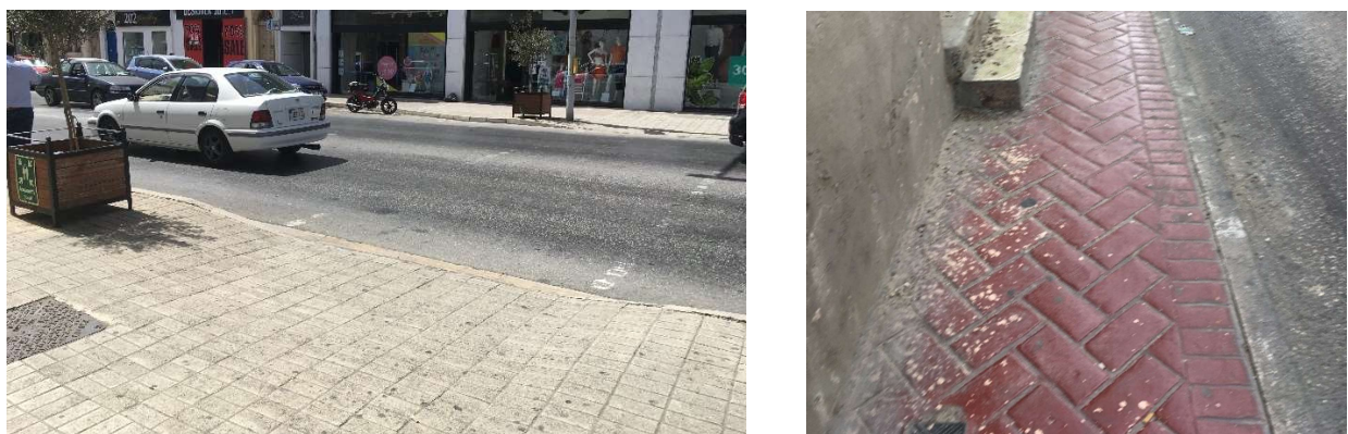
Figure 54: Ramps without blister paving (left) and slippery paving (right). Both scored as 'not suitable materials'
