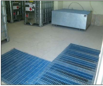
Solvent Storage with secondary containment, fire detection
