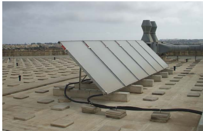
Installation of Solar Water Heaters supplying hot water to the changing rooms
