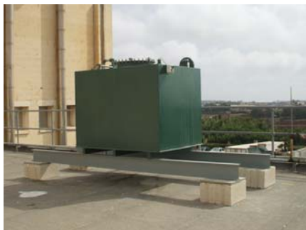
Replacement of Diesel Day Tanks to ones with integrated containment complete with level control system and alarms.
