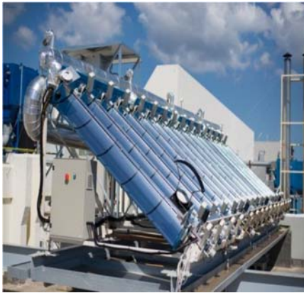
Pilot Project - Generation of Thermal Energy from Solar Power – fed into Factory Steam System
